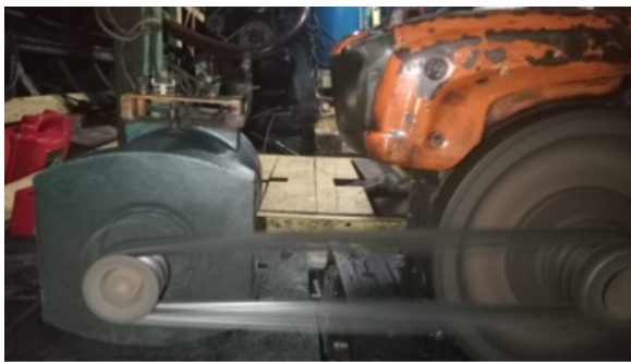
Gambar 3. Mesin generator KM Sena Express
